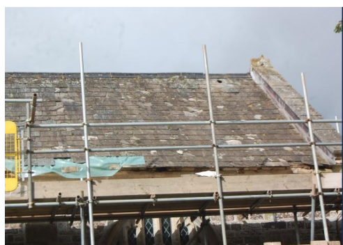
← Multiple slipped roof slates to be replaced.
