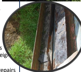
Failed guttering causing interior damp walls. →
